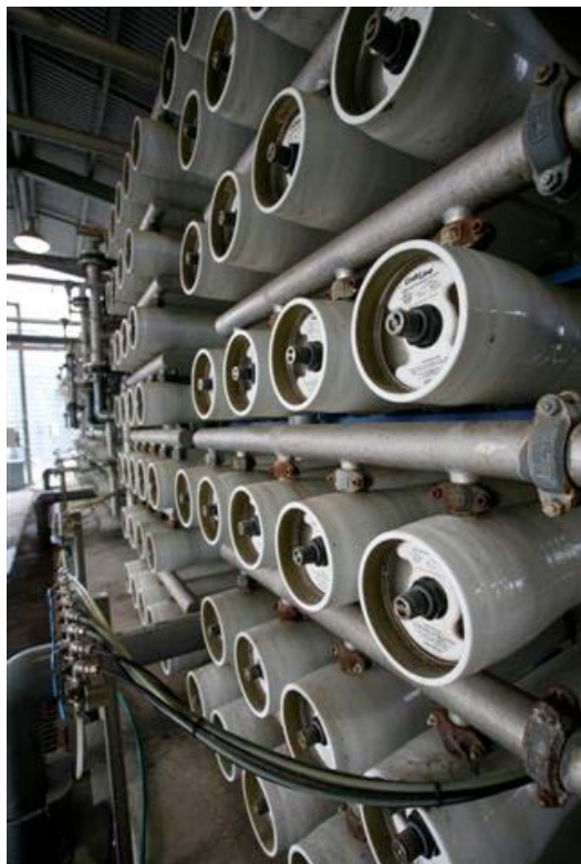
Figure 21 Reverse osmosis – one of the processes used in water purification
