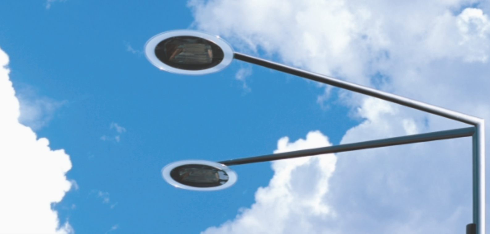
ACTEW supported energy efficient streetlight
