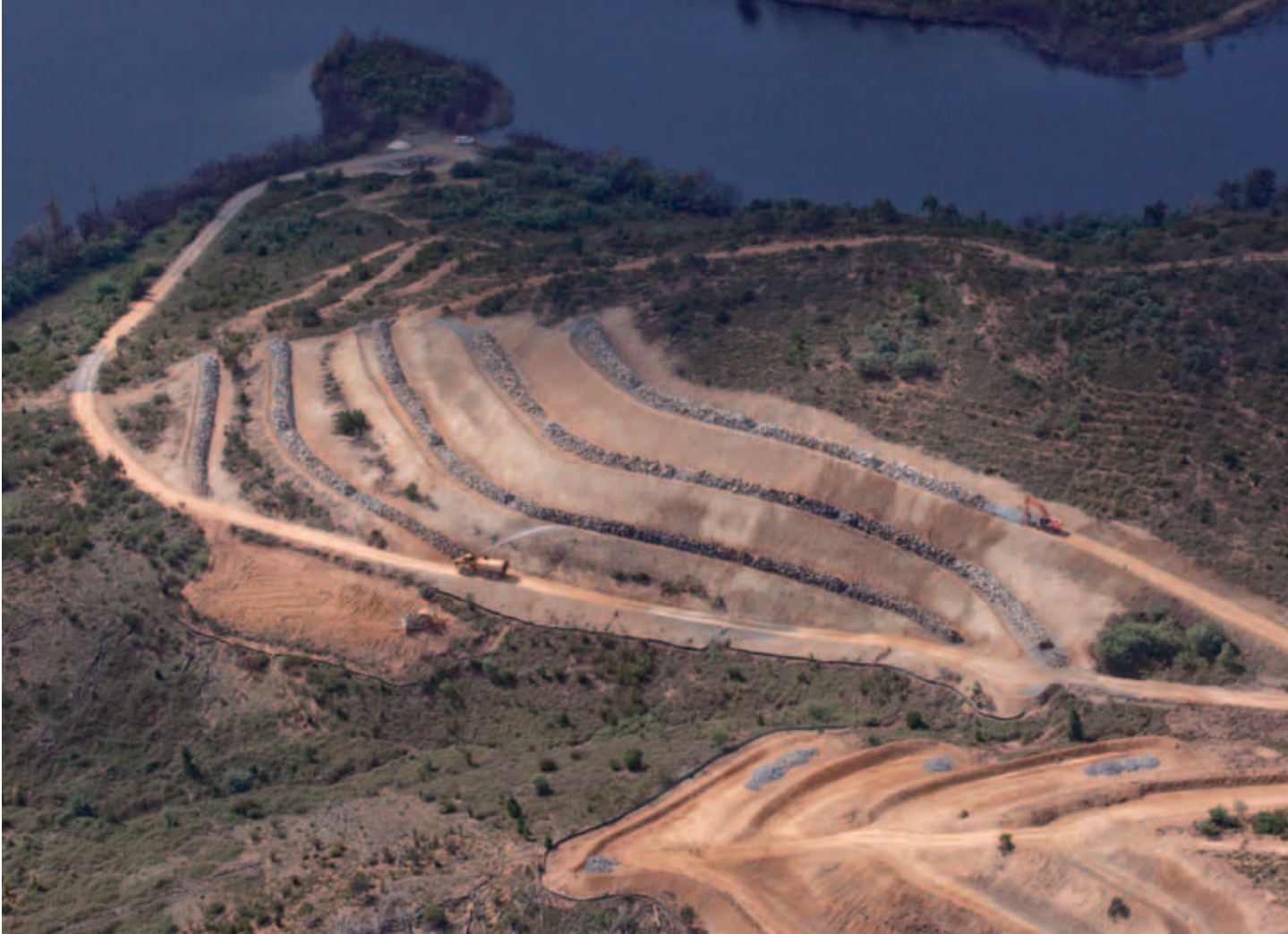
Approximately 4km of fish habitat was constructed in the new Cotter Reservoir inundation area to protect the endangered Macquarie Perch.
