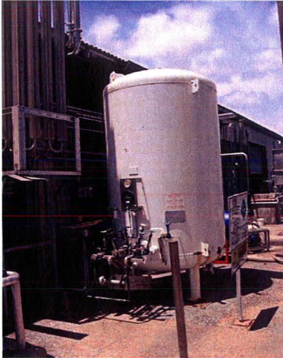
Figure 7 - Photograph of 2.5 tonne refrigerated CO 2 storage vessel (courtesy BOC Gases)
