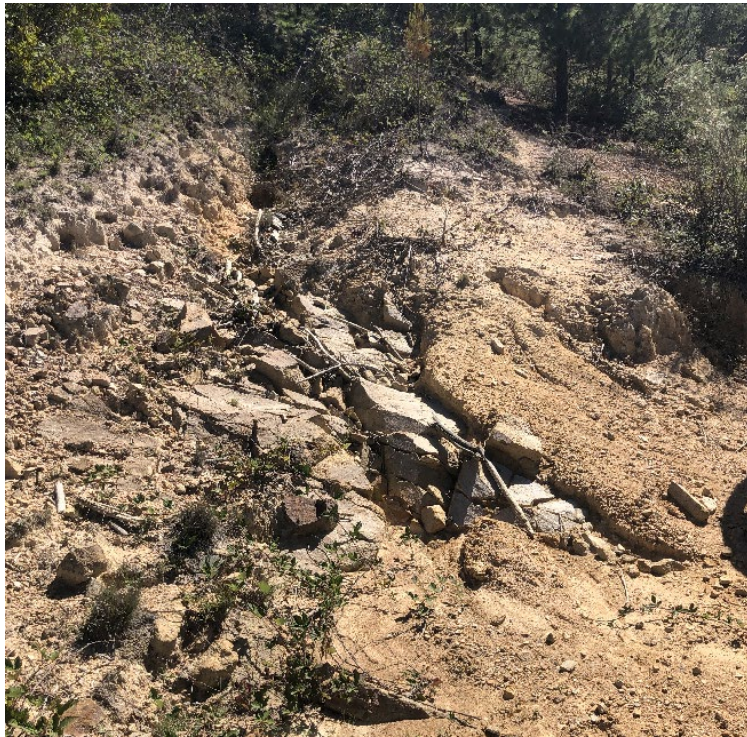
Site MZ7. Rill erosion along the disused track downstream of the shown in the image to the right.
