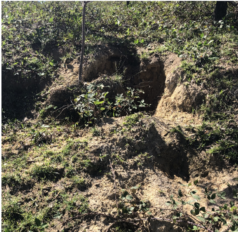
Site MZ4a slumping at radial head cut toward the upper end of the gully
