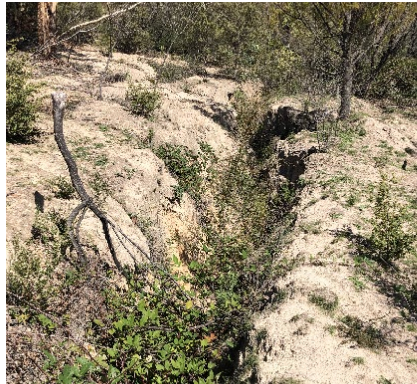
Site MZ1a: Approx. 2m deep incision along contour banks downstream of East West Break road crossing
