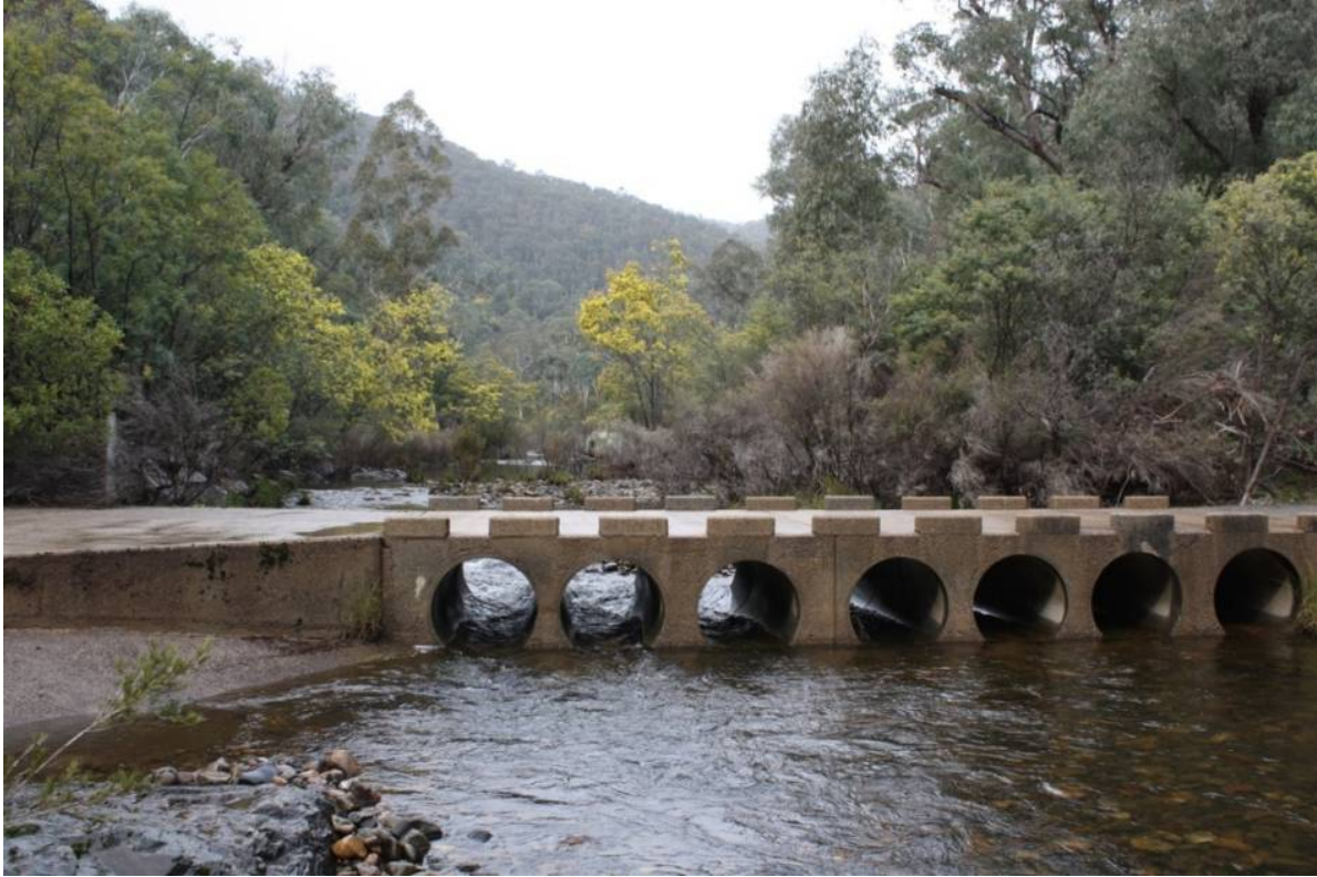
Plate 5 - Pipeline Crossing prior to remediation
