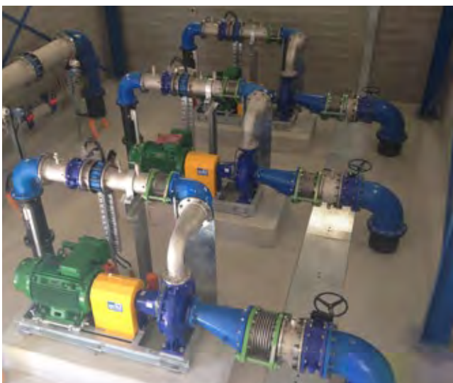
Googong Township Pump Station
