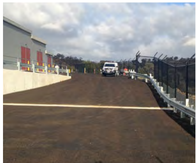
Hardstand area at Googong Township Pump Station
