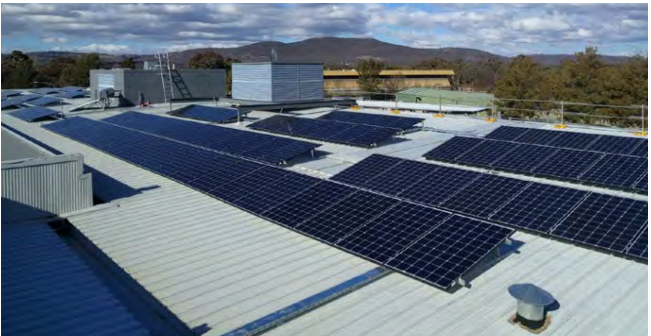
Solar PV Panels at Mitchell office
