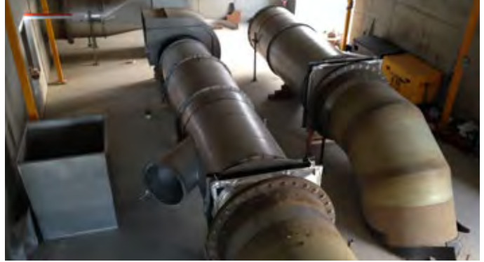
Ventilation ducting manifold
