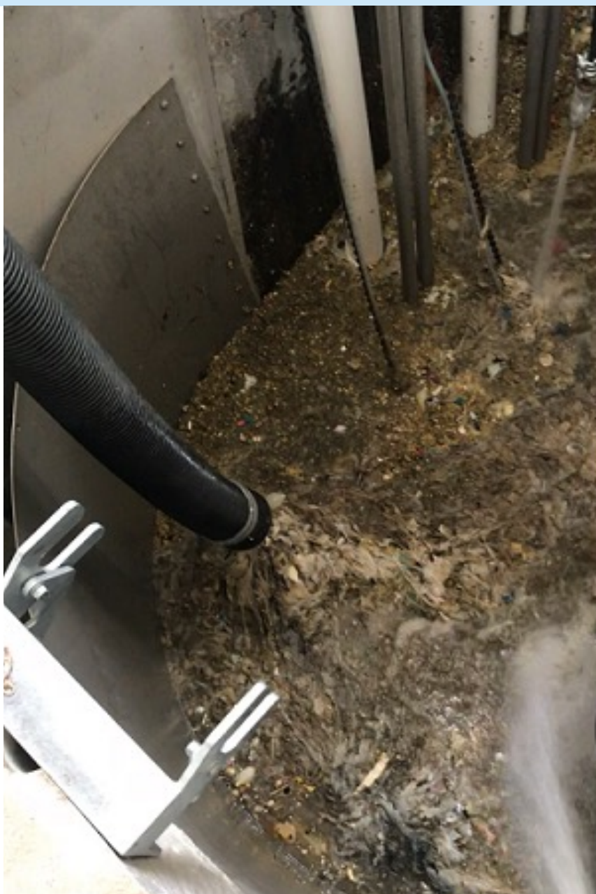
^ View looking down at Temporary Screenings Wet Well, removing wet wipes to minimise pump blockages.
