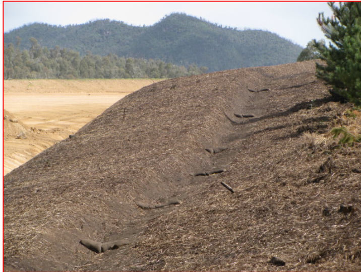
Figure 5.1 Typical hydromulching application along a drainage line and its verge using straw mulch and bitumen.
