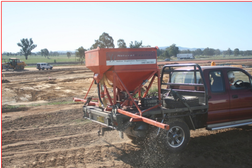
Figure 5.5 Air seeding on a major road infrastructure project in the South West Slopes of NSW (Photo courtesy of Natural Capital).
