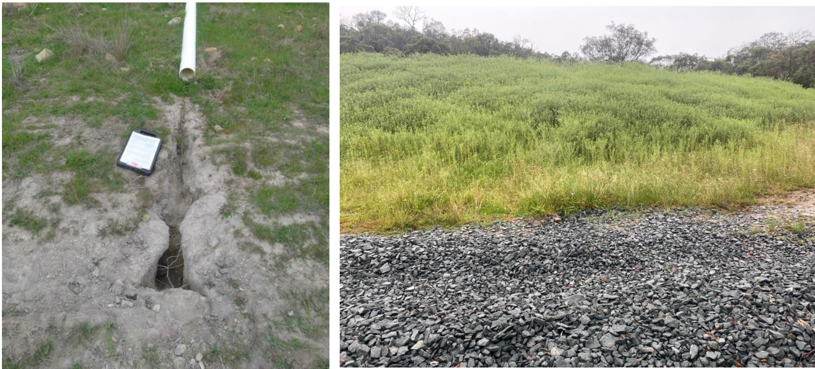
Figure 39: Erosion point 22; as observed during baseline surveys in 2013 (left) and in 2020 (right)
