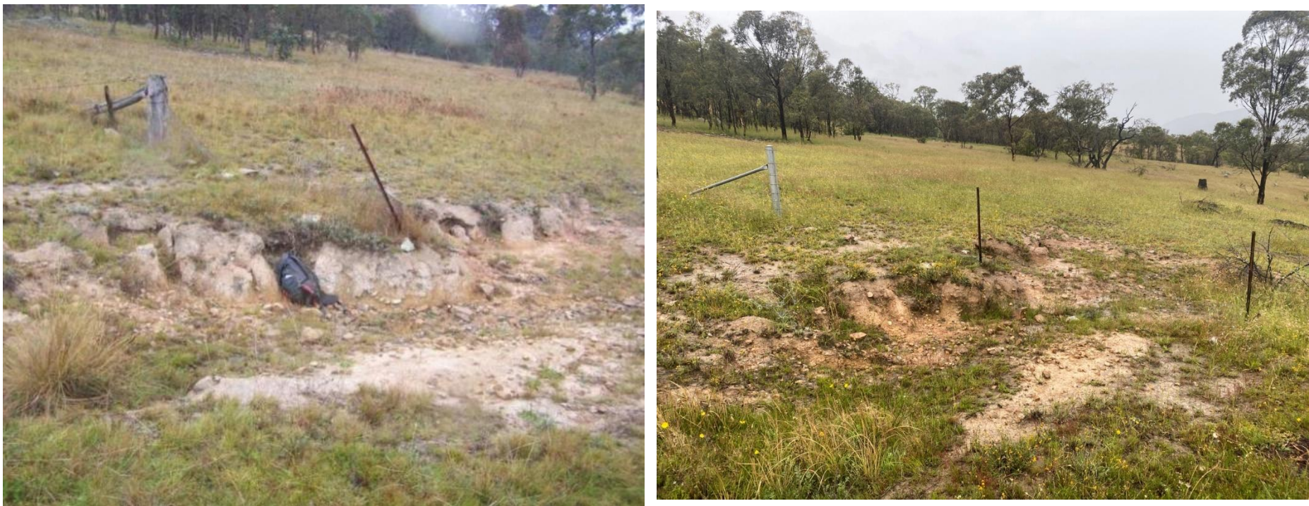
Figure 35: Erosion point 10; as observed during baseline surveys in 2012 (left) and in 2020 (right)
