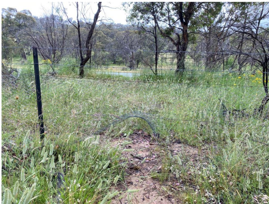
Figure 41: Example of low risk damage to fence where rabbit netting is forced up and becomes a run for animals. Eastern boundary fence, MU3
