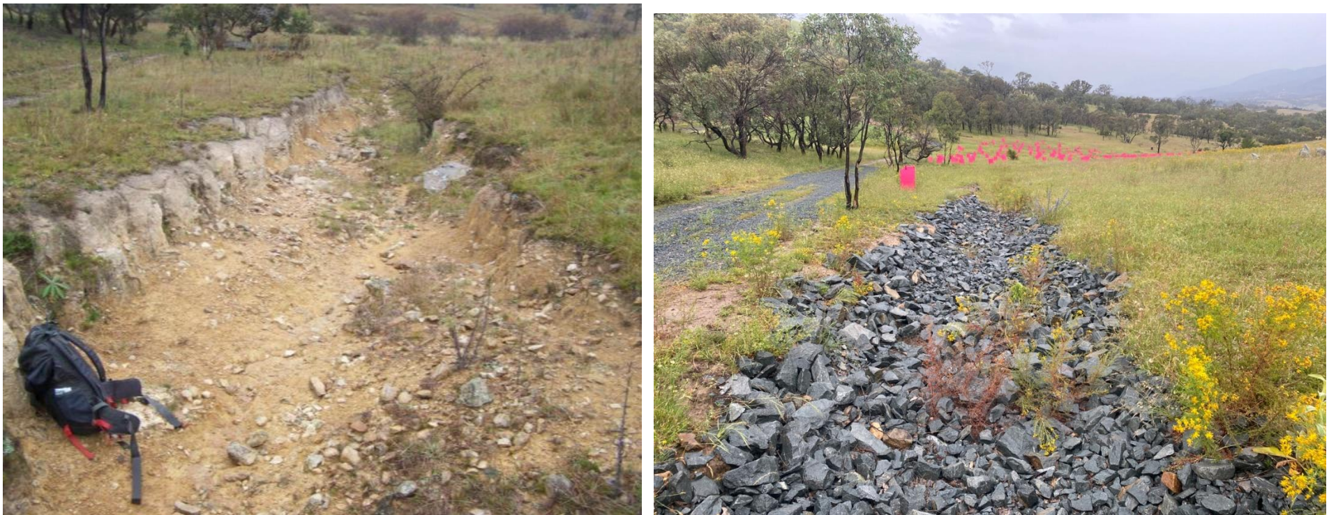
Figure 34: Erosion point 9; as observed during baseline surveys in 2012 (left) and in 2020 (right)
