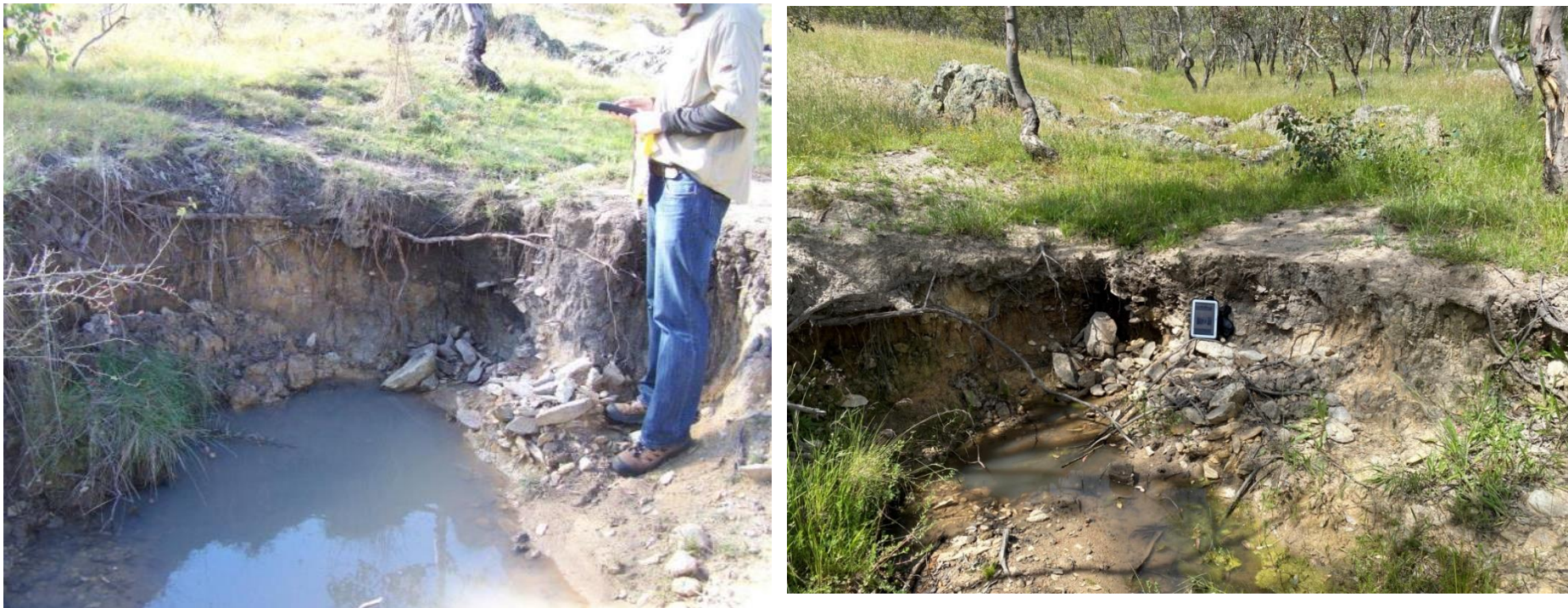
Figure 36: Erosion point 13; as observed during baseline surveys in 2012 (left) and in 2020 (right)
