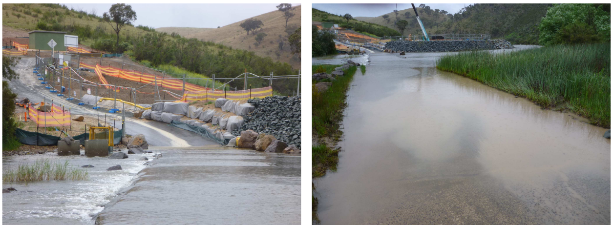
Plate 5. Runoff from the unsealed road at Angle Crossing South side (left) and north side (right)
