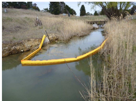
Silt boom downstream of Williamsdale Bridge
