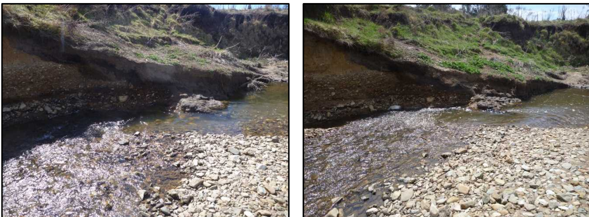
Photo 2 - High erosion potential area downstream of Pool 5 during September (left) and October (right) 2012
