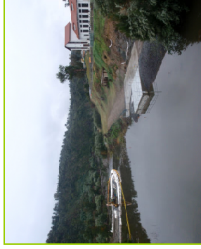
A view looking downstream of the bridge with sediment control structure and MPS
