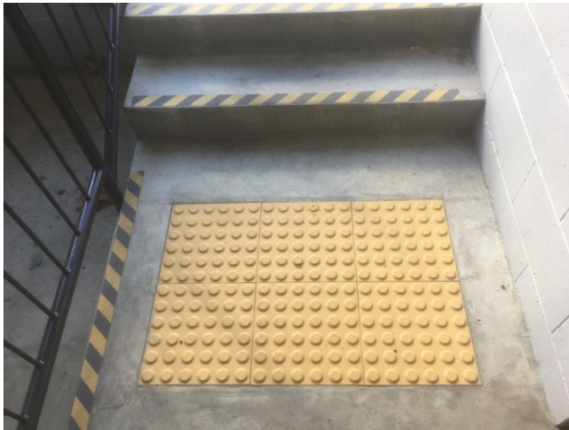
Fig. 5.13.1.1 Proprietary anti-slip tiles embedded within a stairway landing
