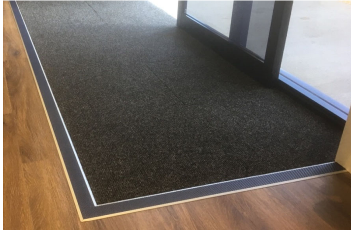
Fig. 5.13.3.1 Edge bevelling of a surface differential (i.e. floor mat) in a doorway
