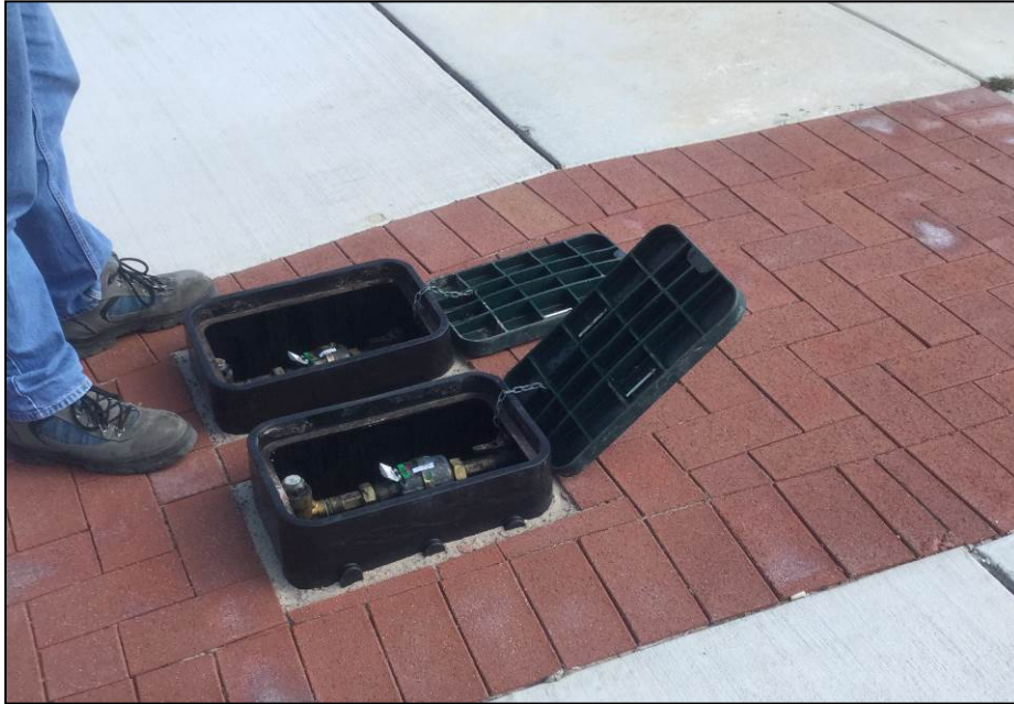
Fig. 8.3 Failed DN20 Water Meter Installation (Water meter and meter box too high)
