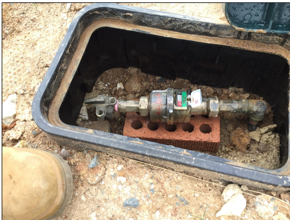
Fig. 8.1 Failed DN20 Water Meter Installation (Not centred; PE100 riser downstream)
