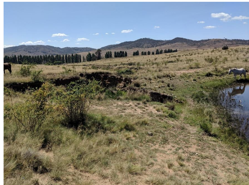
Failing dam embankment looking east
