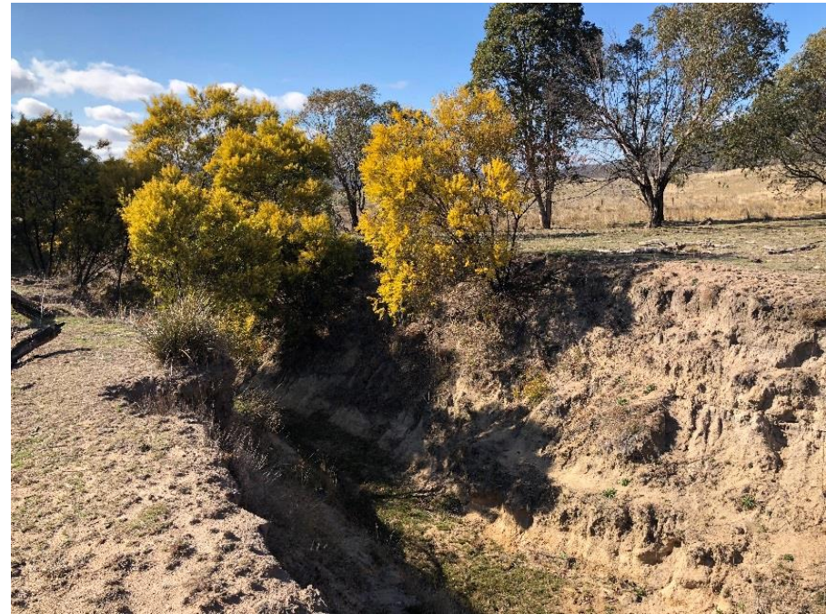
Bank erosion along Spring Station Creek
