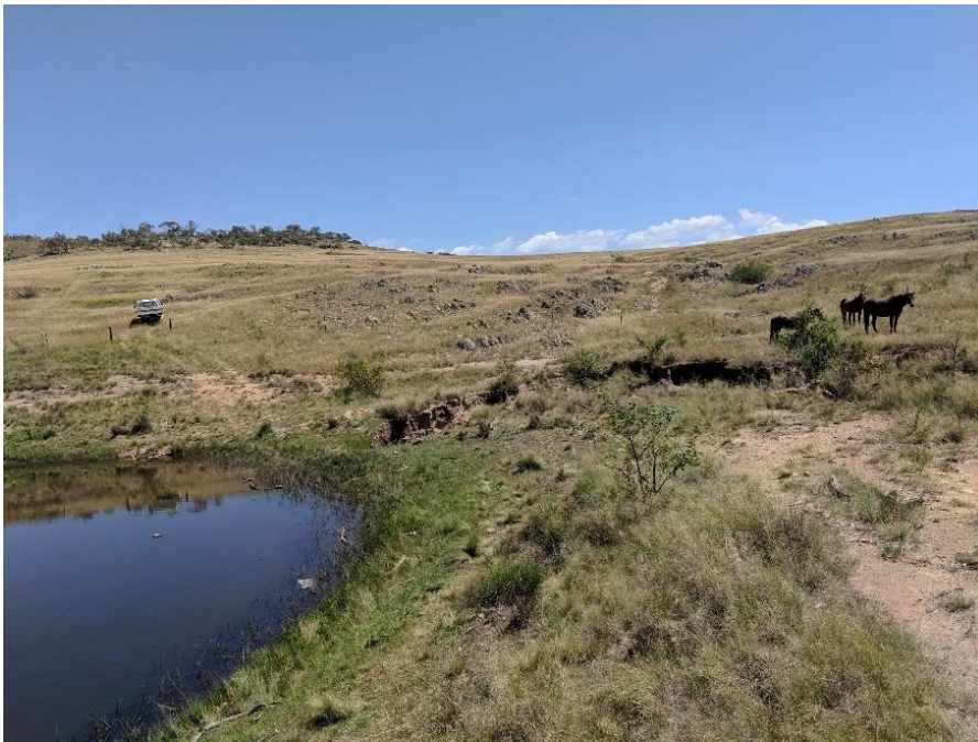
Failing dam embankment looking west
