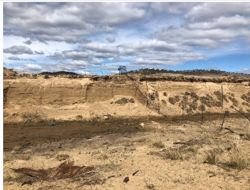
Banks with isolated slumping
