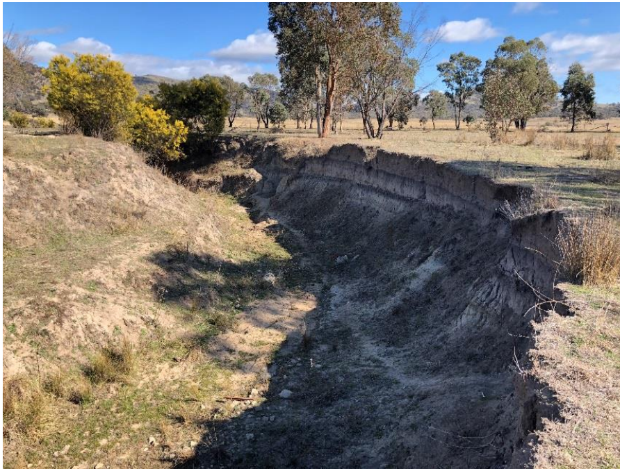
Bank erosion just upstream of the gully's confluence with Spring Station Creek
