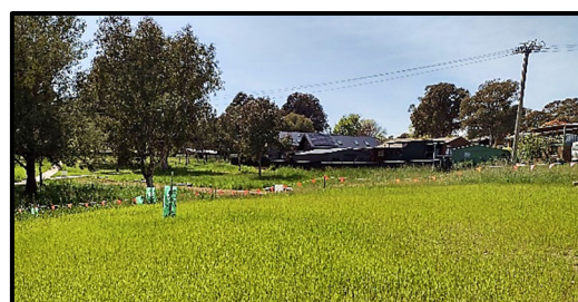
Restoration work across the pipeline corridor is expected to be completed by April 2023, weather permitting.
