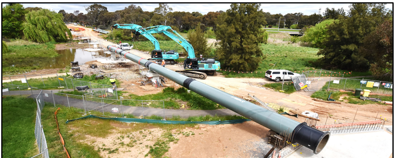
Excavators use slings to lift the 12-ton sections of pipe to form the pipe bridge cross Ginninderra Creek.
