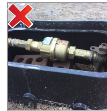
Incorrect meter height
