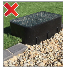
Incorrect box level
