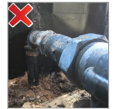
No copper risers
