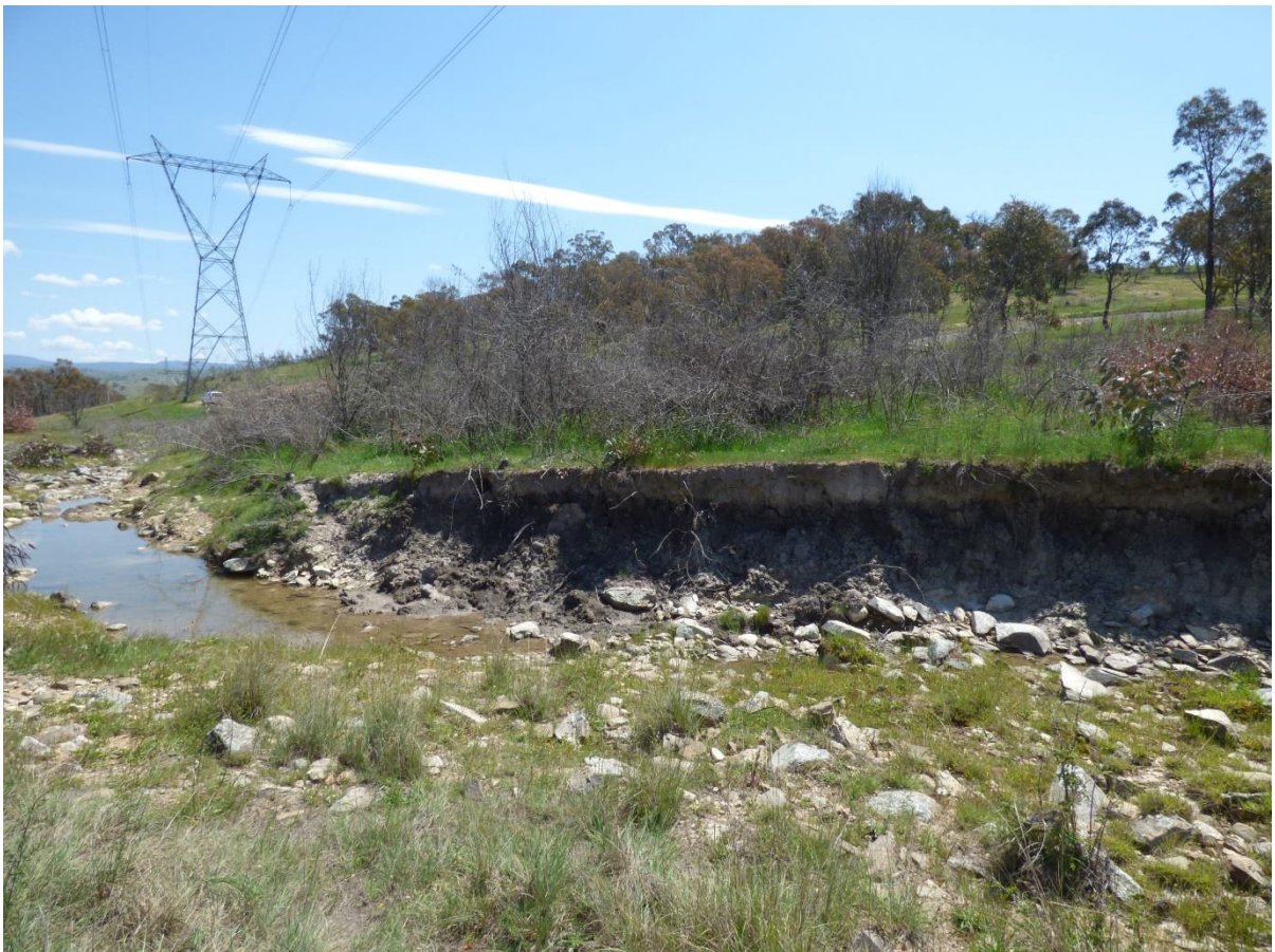
Figure 18 Erosion occurring along main drainage line, northern offset
