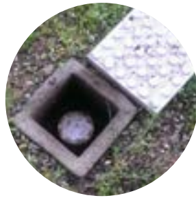
Riser or inspection shaft
