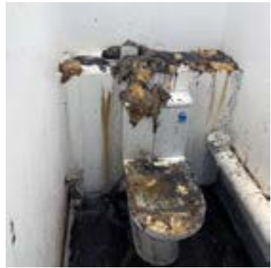
Result of customer blockage
