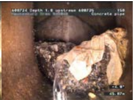
Wipes clumped in a concrete pipe
