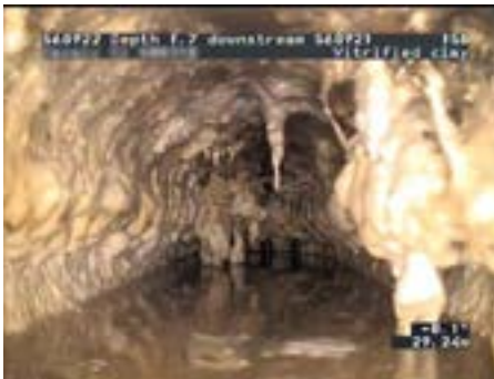
Build up and clogging of pipes
