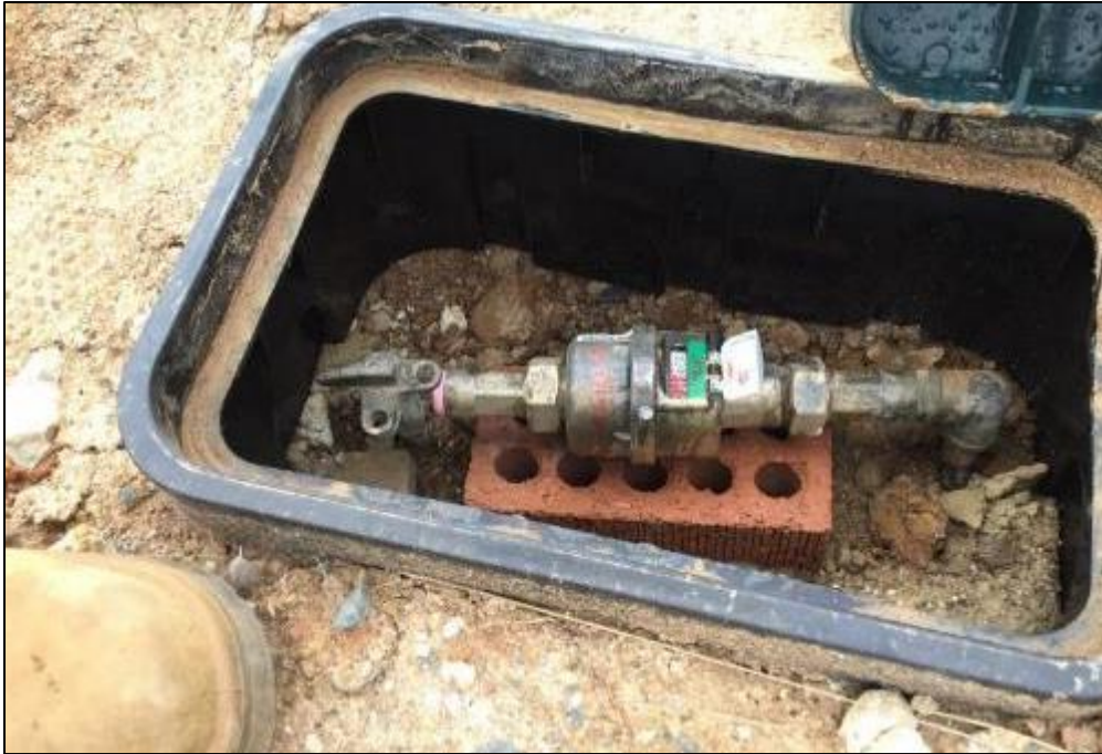
Fig. 8.1 Failed DN20 Water Meter Installation (Not centred; PE100 riser downstream)
