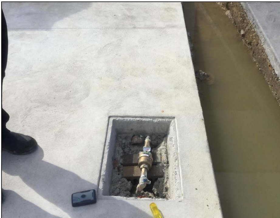
Fig. 8.4 Failed DN20 Water Meter Installation (Water meter in driveway and meter too high)
