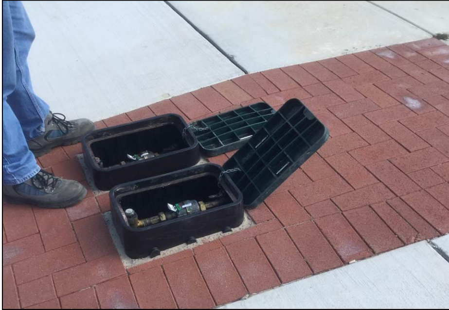
Fig. 8.3 Failed DN20 Water Meter Installation (Water meter and meter box too high)
